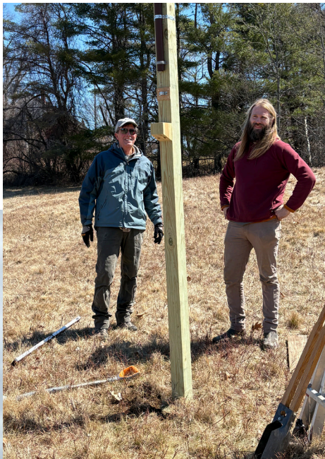
MCA board member Alan Phipps and project leader Logan Parker are happy to have finished installing the support pole at the Salt Bay Farm box. (Jeff Cherry photo)
